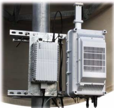
C-Band High power Block Up Converter system
